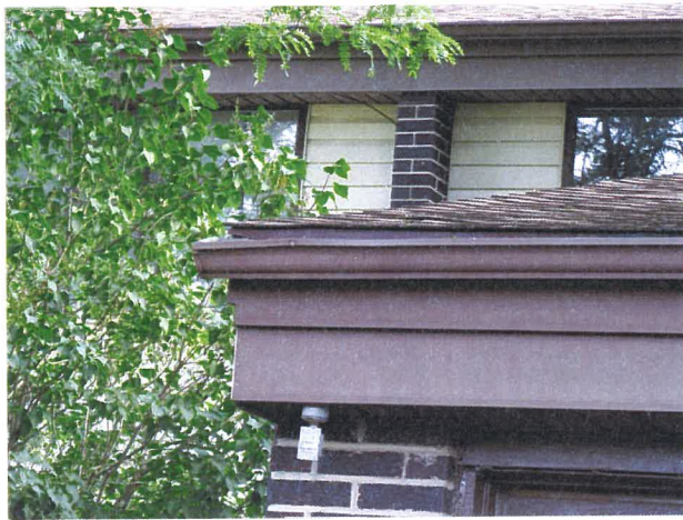
Gutter damage noted at Unit 1004
