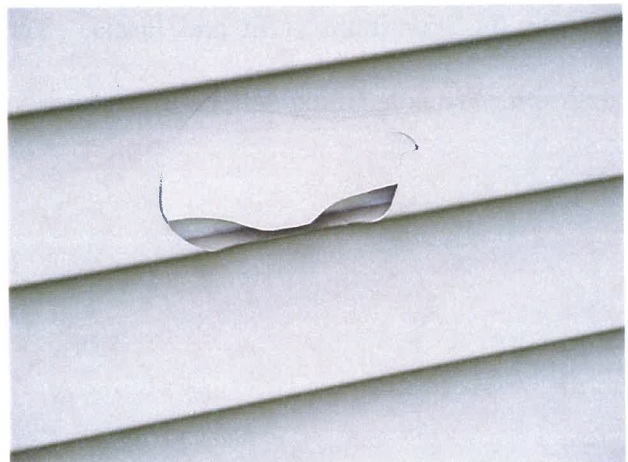
Garage siding damage noted at Unit 454
