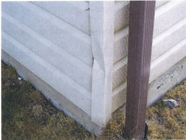
Aluminum trim damage noted at Unit 1406
