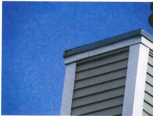
Chimney cap corrosion noted at Unit 1604
