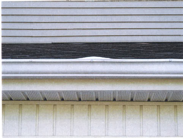
Gutter damage noted at Unit 1601
