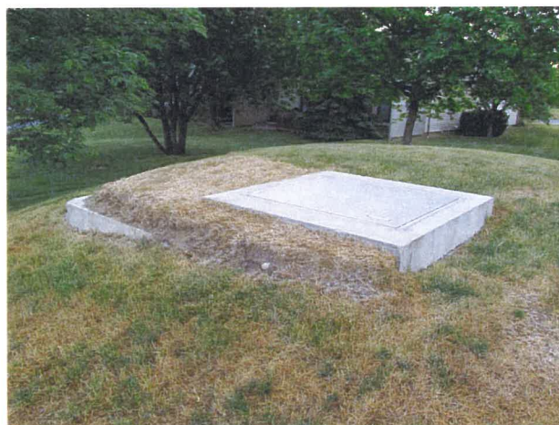
Water main backflow prevention valve structure
