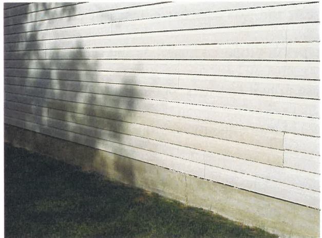
Non-uniform siding color noted at Unit 1108
