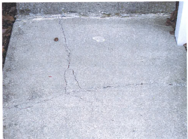
Concrete sidewalk cracks
