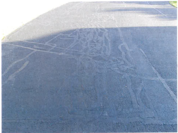
Significant crack repairs
