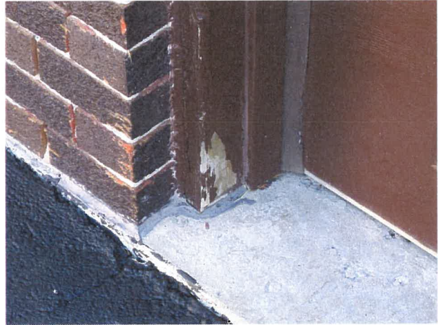
Garage trim paint deterioration noted at Unit 1304
