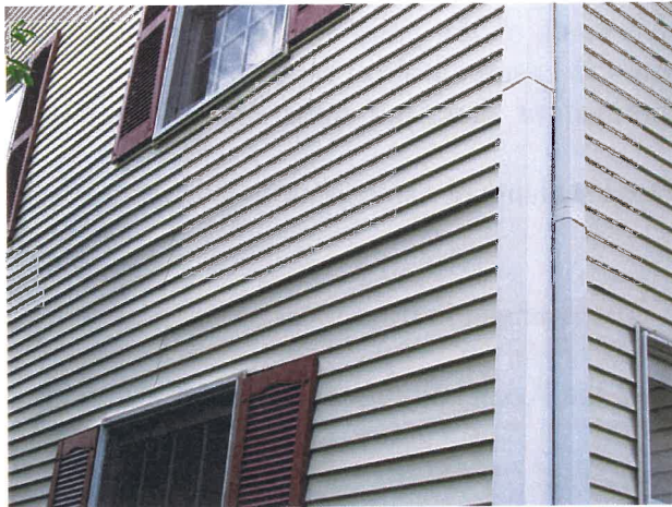
Siding deflection noted at Unit 103
