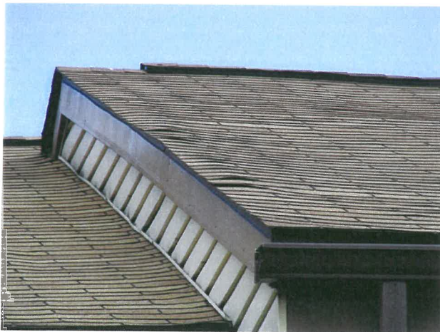
Shingle lift noted at Unit 855
