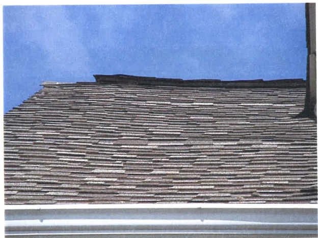
Ridge vent deflection noted at Unit 703
