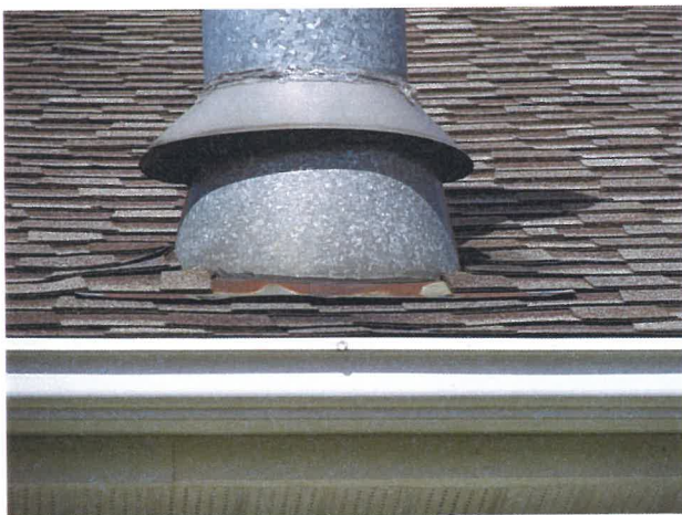
Waste pipe flashing corrosion noted at Unit 453
