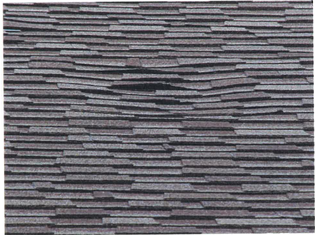
Sheathing deflection and shingle lift noted at Unit 153
