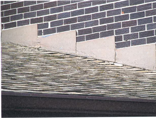
Flashing finish deterioration noted at Unit 1054
