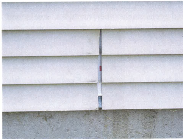
Siding gap noted at Unit 206
