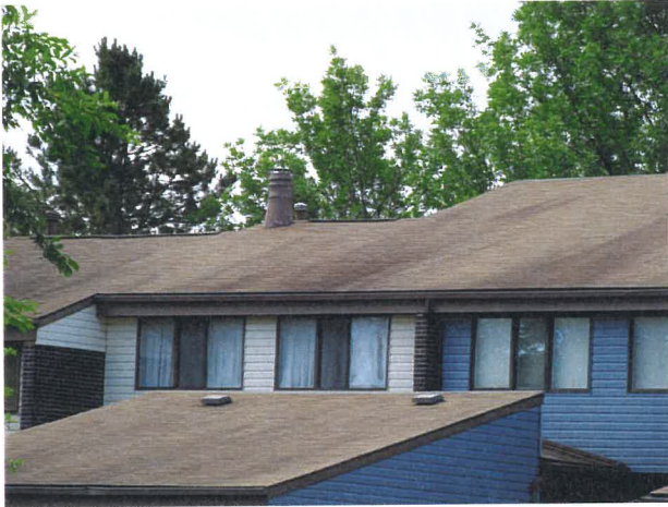
Streaking noted at building containing Units 951 through 958
