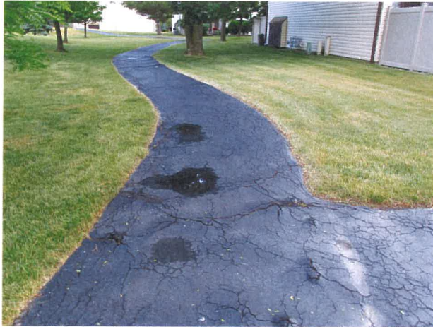
Asphalt pavement walking path overview, note significant cracking
