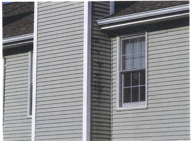
Typical siding stains from gutter overflow
