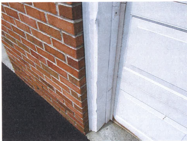
Garage door trim damage noted at Unit 312
