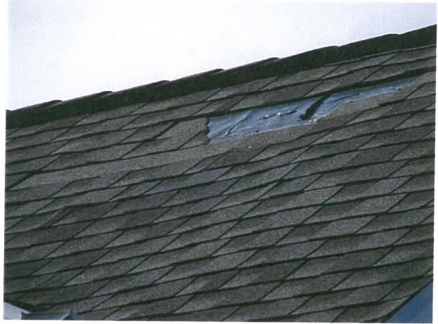
Missing shingles noted at Unit 1603
