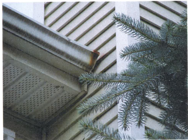
Gutter corrosion noted at Unit 301
