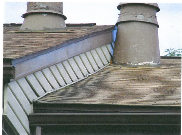
Granular loss noted at Unit 853
