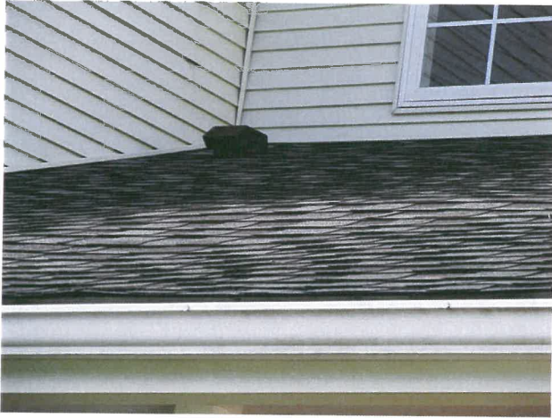
Sheathing deflection noted at Unit 1703
