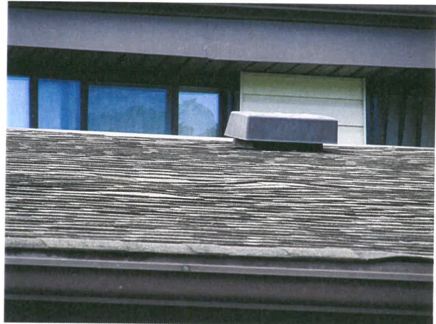
Sheathing deflection noted at Unit 752
