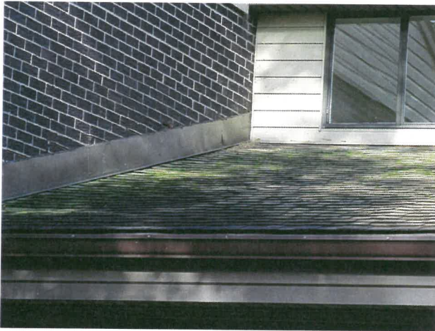
Organic growth noted at Unit 1501
