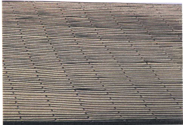
Curled shingles noted at Unit 953
