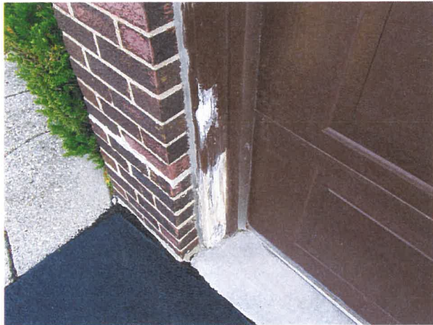
Garage trim paint deterioration noted at Unit 806
