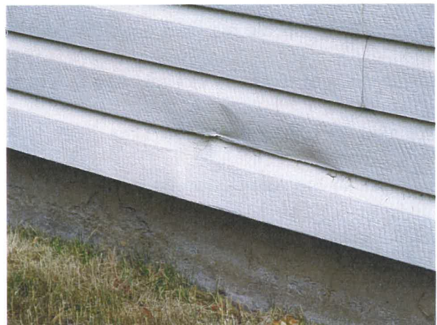
Siding damage noted at Unit 1151
