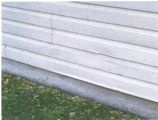
Siding damage noted at Unit 754
